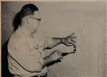
When light switches or other equipment in the ward house need repairing, Brother Stoll is the one who does the job.
